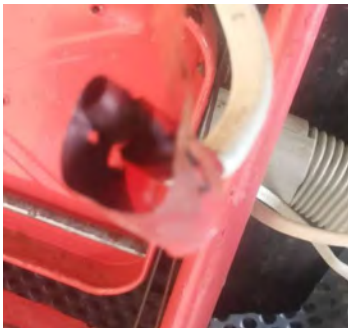
Exposed Live Conductor
